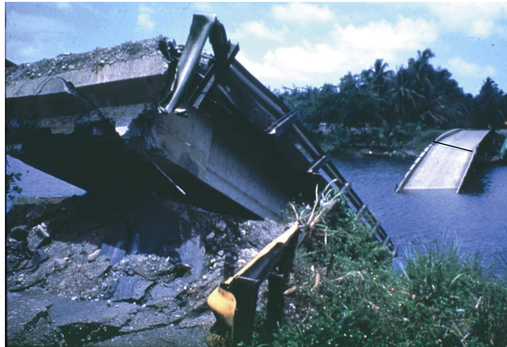
Skewed bridge pushed off of supports due to lateral spread displacements in 1991 Costa Rica Earthquake
