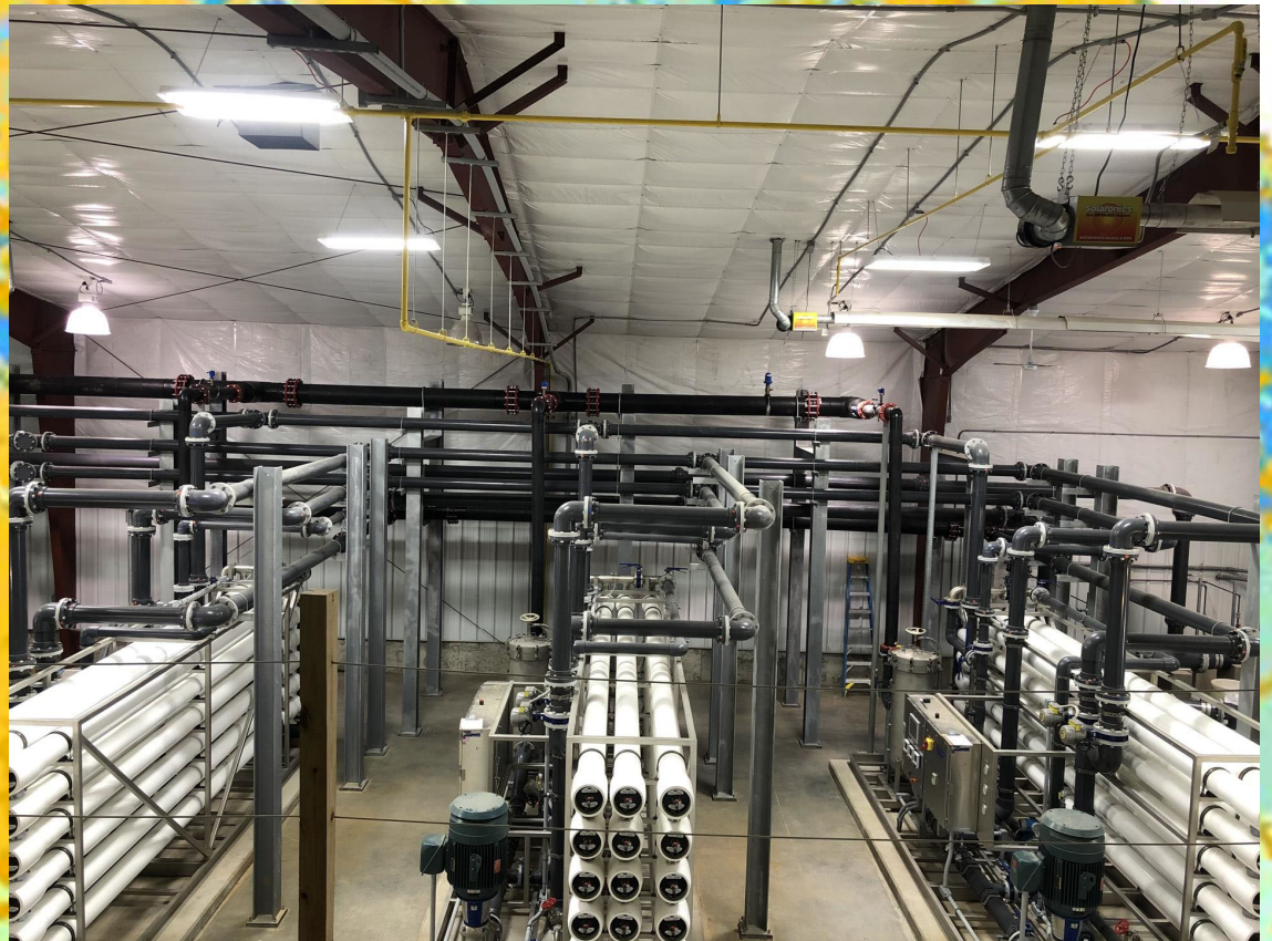
Water filtration system, Lakin, KS
